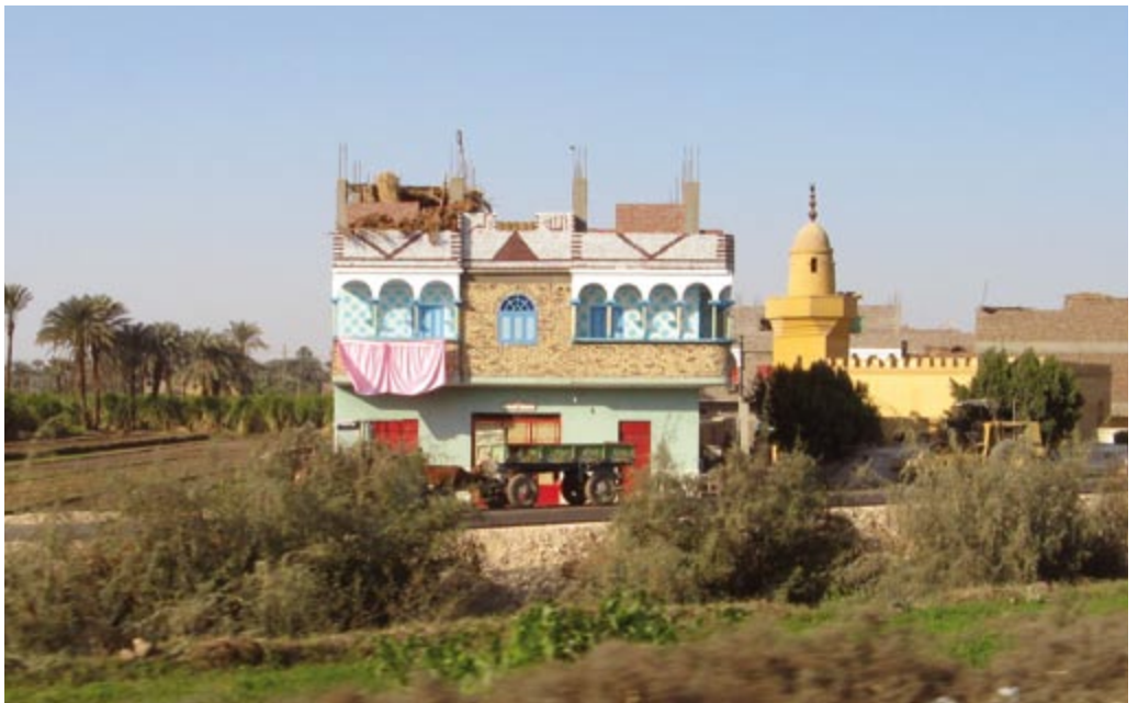
p. 123 - Bare rebar crenellations rise from the roofs of most concrete buildings
